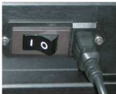
Figure 6-2 Main power switch and cable
