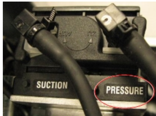
Figure 6-126 Tubes connected to the waste pump
